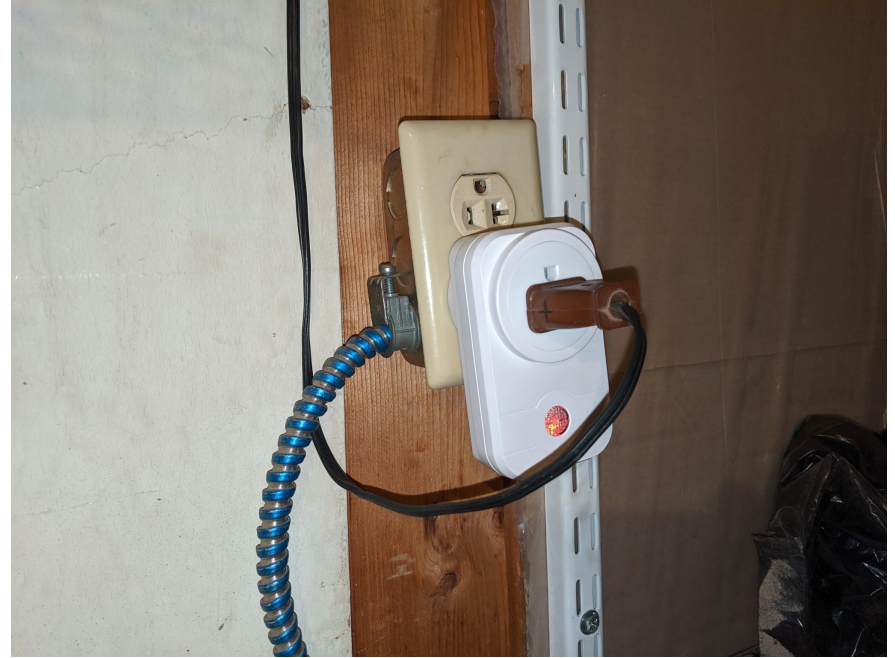
Using a smart relay to control garage light.
