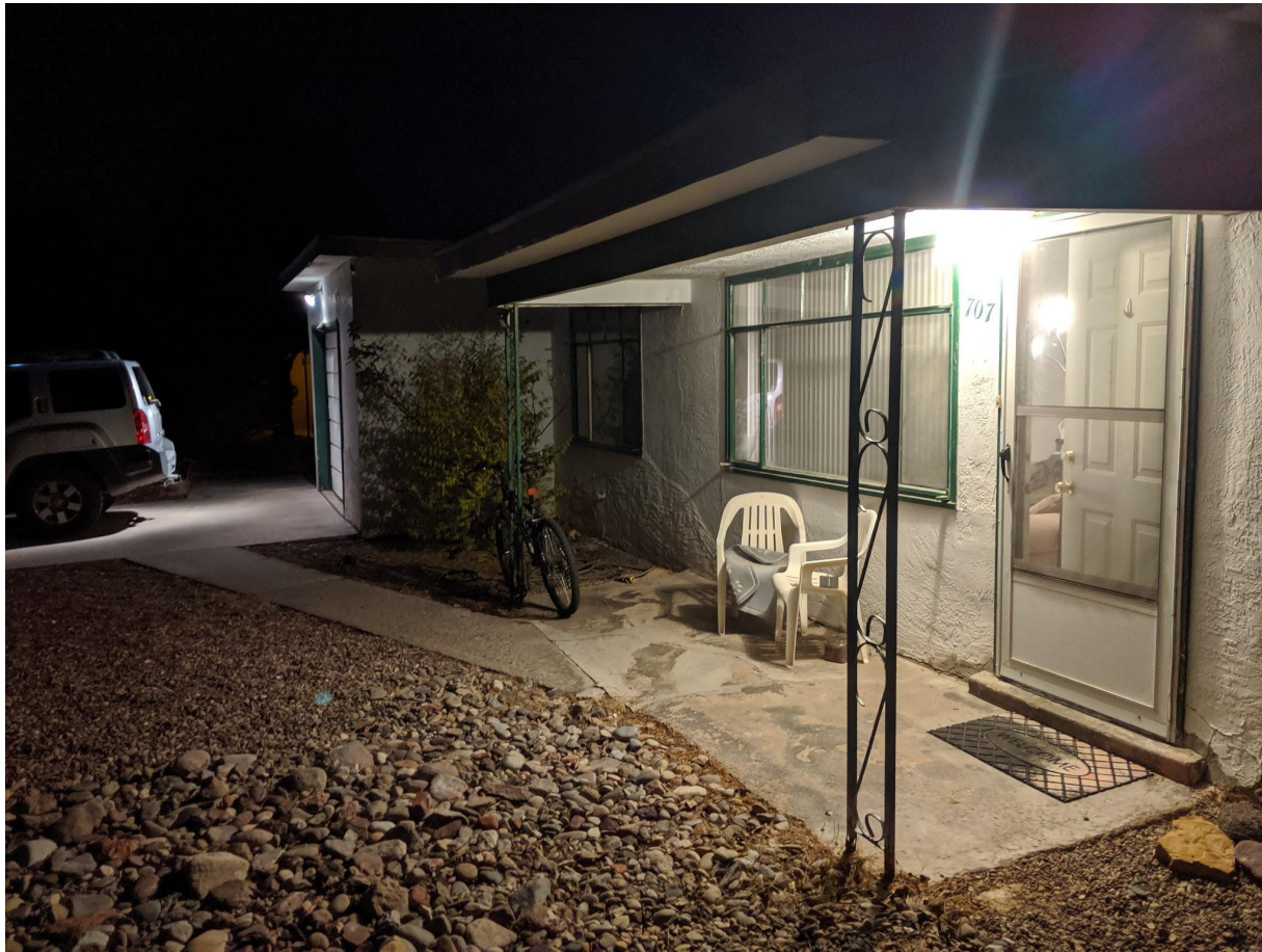
The separation between the front door and the garage. Using the switch and relay together allows the front yard to be illuminated more evenly.
