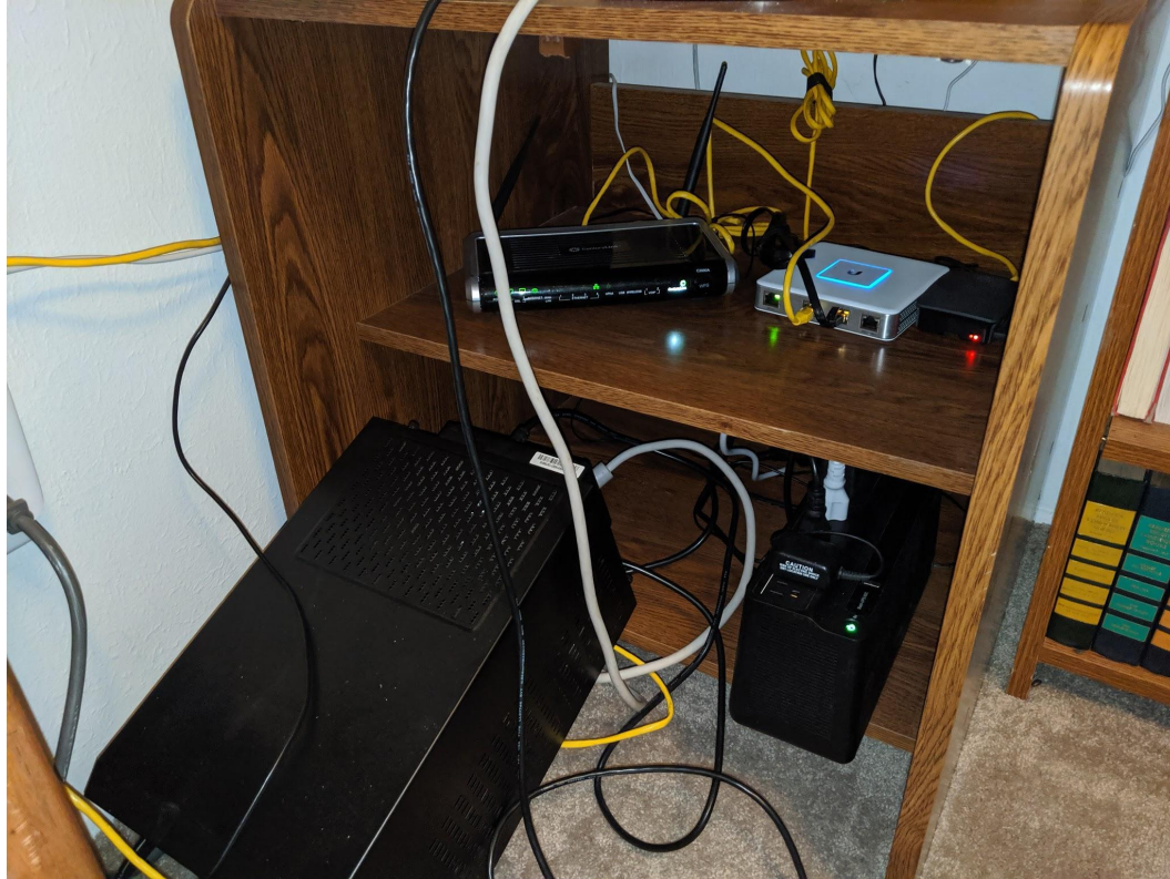
The guest server room current status after a boot issue fix.
