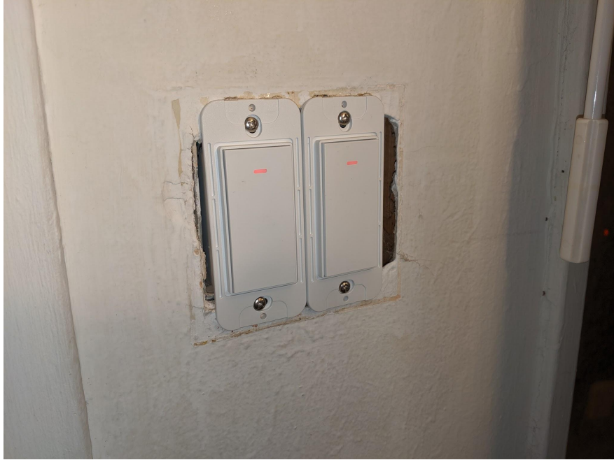
Smart switches installed inside the home.
